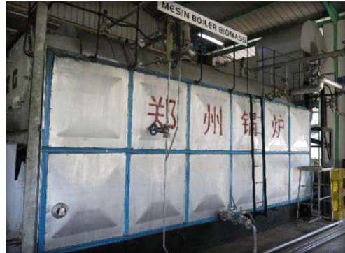
Boiler Biomass Pellet
